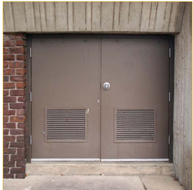
Hollow metal doors require constant maintenance
